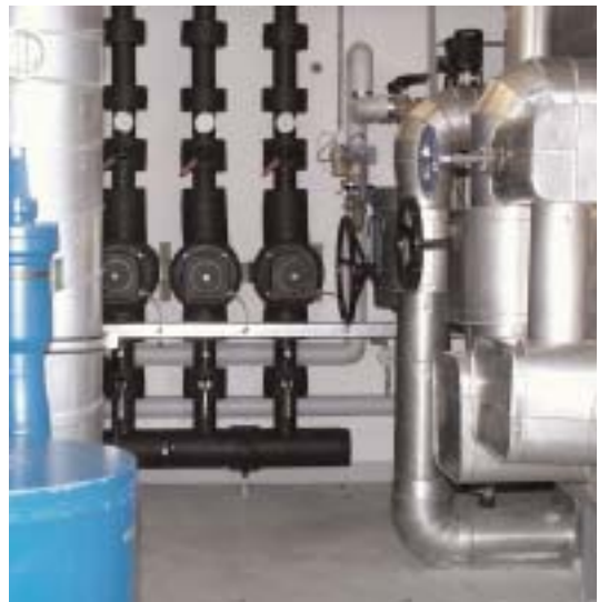
Brine circulating pumps
